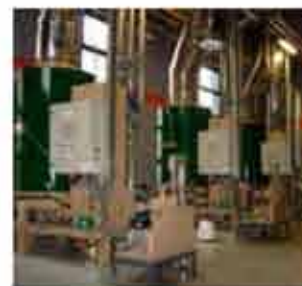
Multiple steam systems
