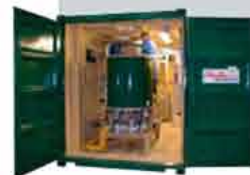
Containerised boiler house
