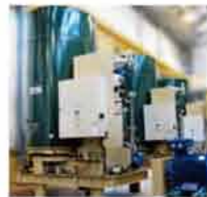
Multiple steam systems
