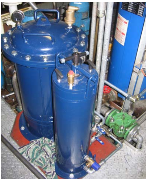
DMA Particle Filter & DMA Absorption Filter installed on-board vessel.
