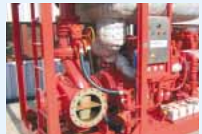
Suctionside of pump
