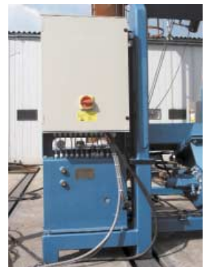
Power pack and control Cabinet
