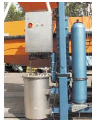
Power pack and control Cabinet
